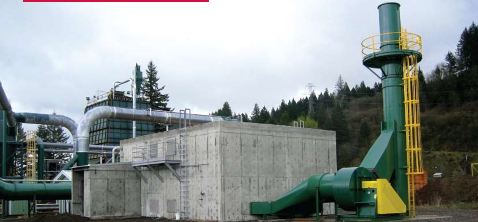
BRI bio-oxidation system on a plywood press
